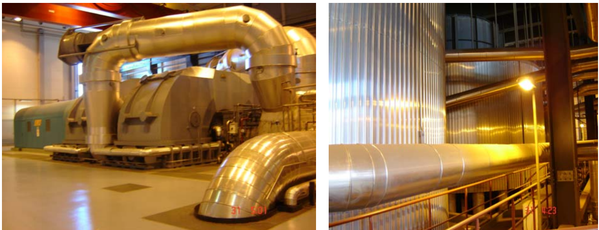
Fig. 5. Turbine hall (left) and cyclones (right) of Alholmens 240 MW power plant
